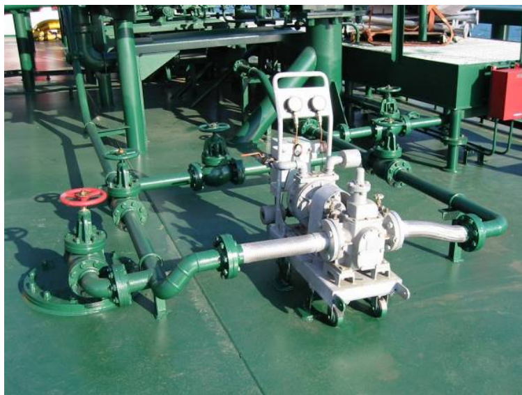
Figure 6 - Midship pumping arrangement at manifold
