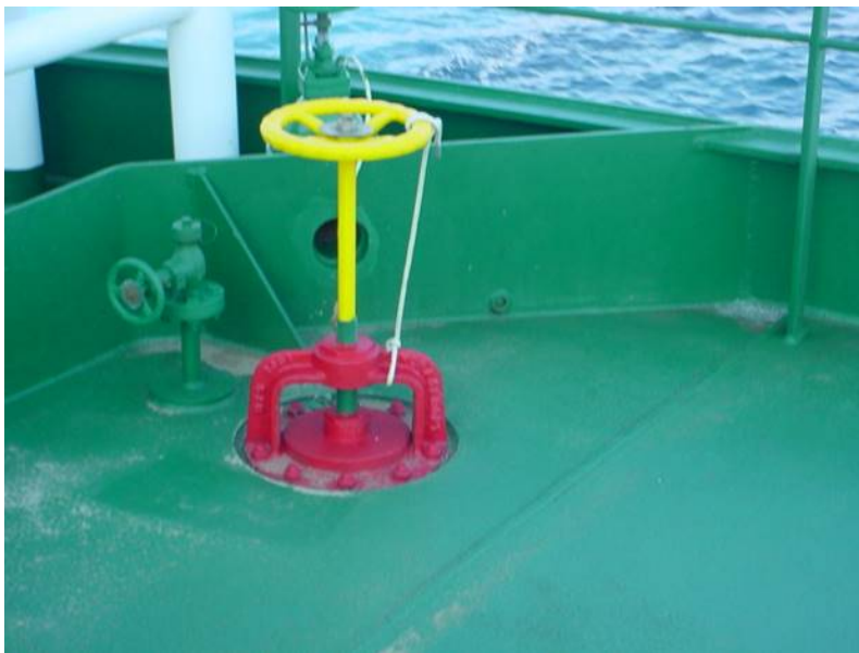
Figure 3 – Deck oil spill dump valve.
